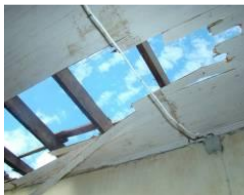
Figure 61 Damages to Post Office Facilities
