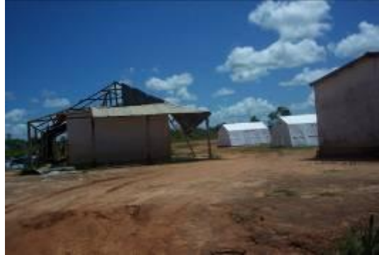
Figure 10: Heavily damaged CEG (middle school) at Besalampy and temporary schools set up in Melaky region
