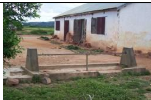
Figure 12: Non-functioning water point at a primary school (EPP) in the Amparafaravola school district
