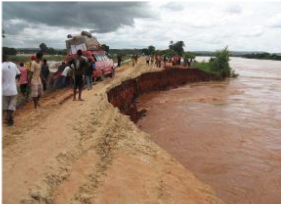
Figure 55 : Erosion of dikes
