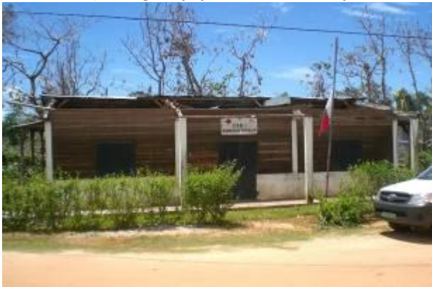
Figure 83: Basic Health Center 1 at Ambodiforaha (Island of Sainte-Marie) damaged by cyclone Ivan, February 2008
