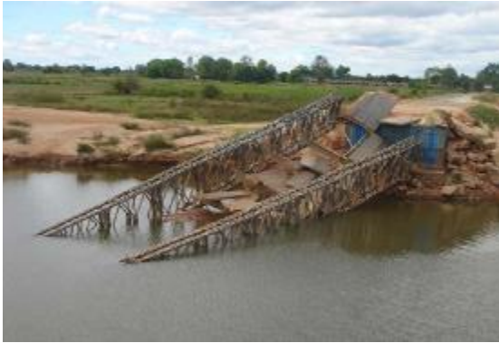
Figure 53 : Overturned bridge on RN 6
