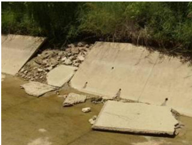
Figure 41: Damage to diversion dike, Menabe region
