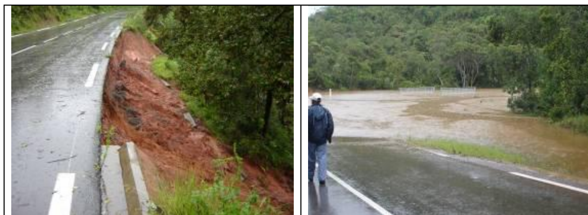
Figure 52 : National Road RN 45: Flooded road and bridge and Breach
