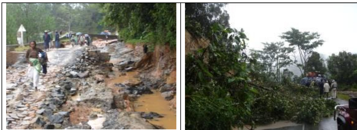
Figure 51 : Damages to RN 25
