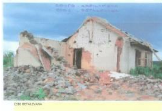
Figure 14: Hospital destroyed by the cyclones
