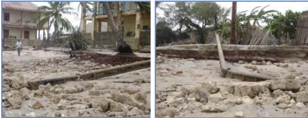
Figure 57: Damage to high-voltage and distribution lines
