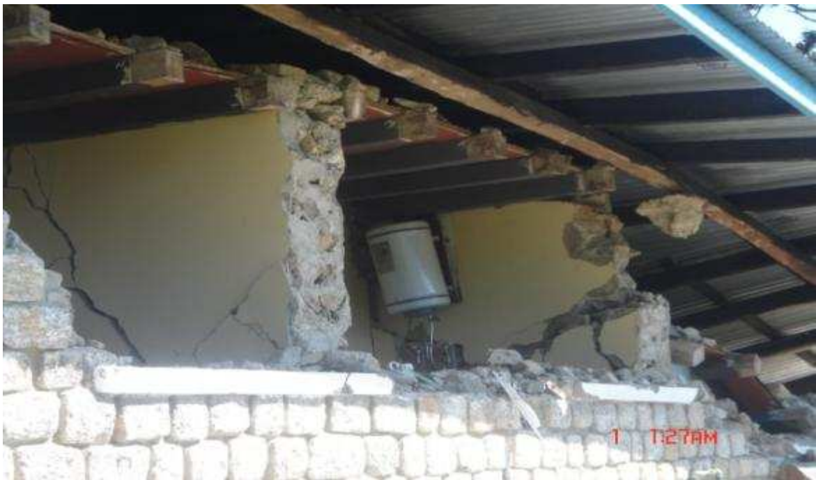
No proper joints between walls
