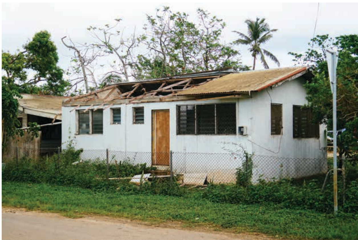
FIGURE 16. A house destroyed by Tropical Cyclone Gita in Longolongo village, Tongatapu, Tonga.
