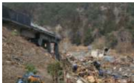
Tracks washed away by the tsunami (Tanohata Village, March 2011)
