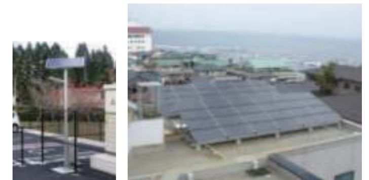
Solar power generator at a daycare center (Noda Village)
