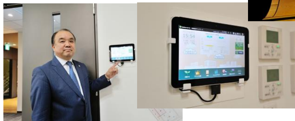
Energy monitor at an office
