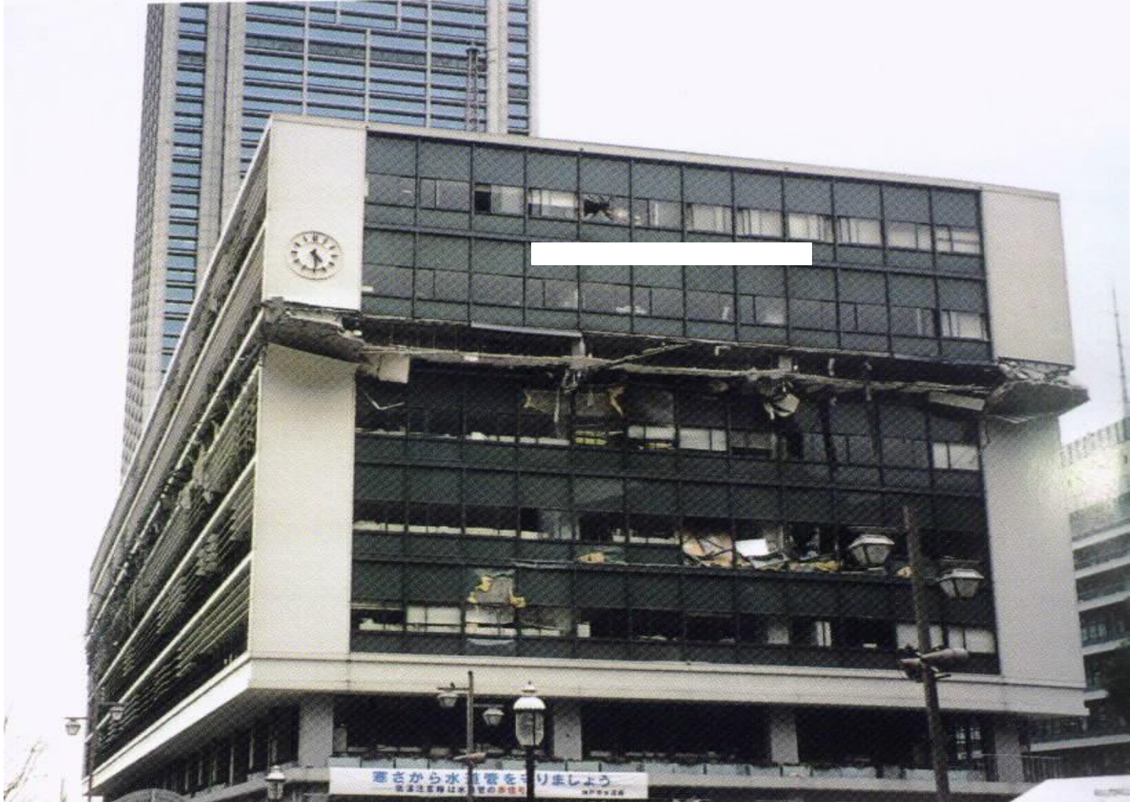
Collapse of the municipal office's mid floors (Chuo-Ward)
