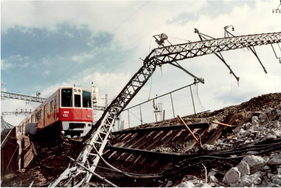
Collapse of Railways (Higashinada Ward)
