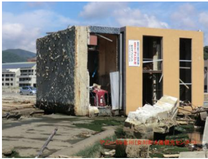
Building that fell down (tipped over) by tsunami
